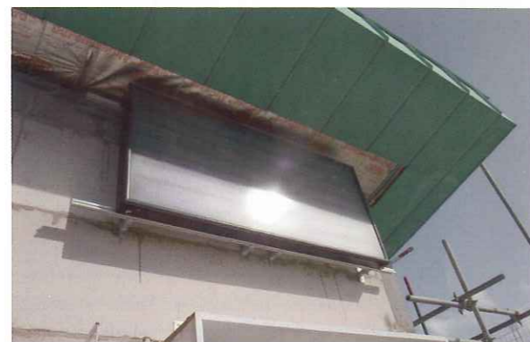
Two solar hot water panels are incorporated in the design
