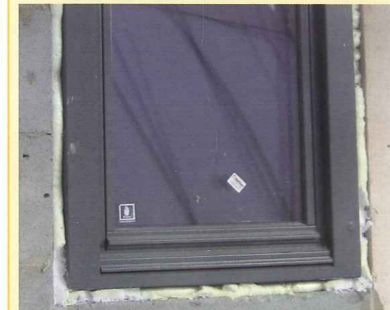
Polyurethane foam was used to create an airtight seal around the windows and doors
