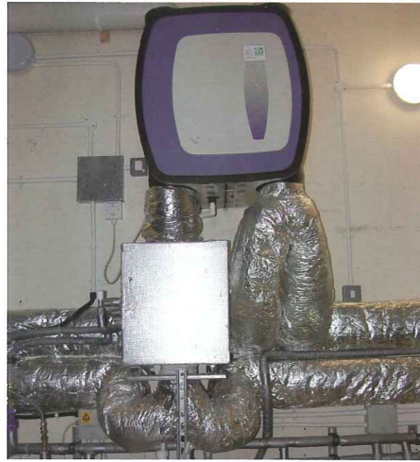
Insulated ductwork to the MVHR unit (by Vortice). The 'post-heater' (small radiator) is located in the metal box and fed by the thermal store (not shown).
